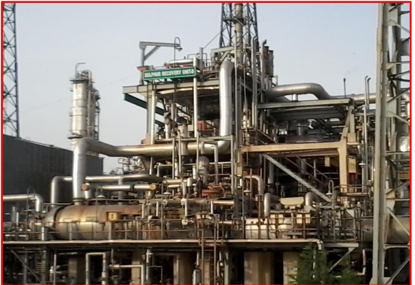
COMPLETION VIEW OF SRU UNIT JOB OF M/S. TECHNIP KT INDIA LTD.
