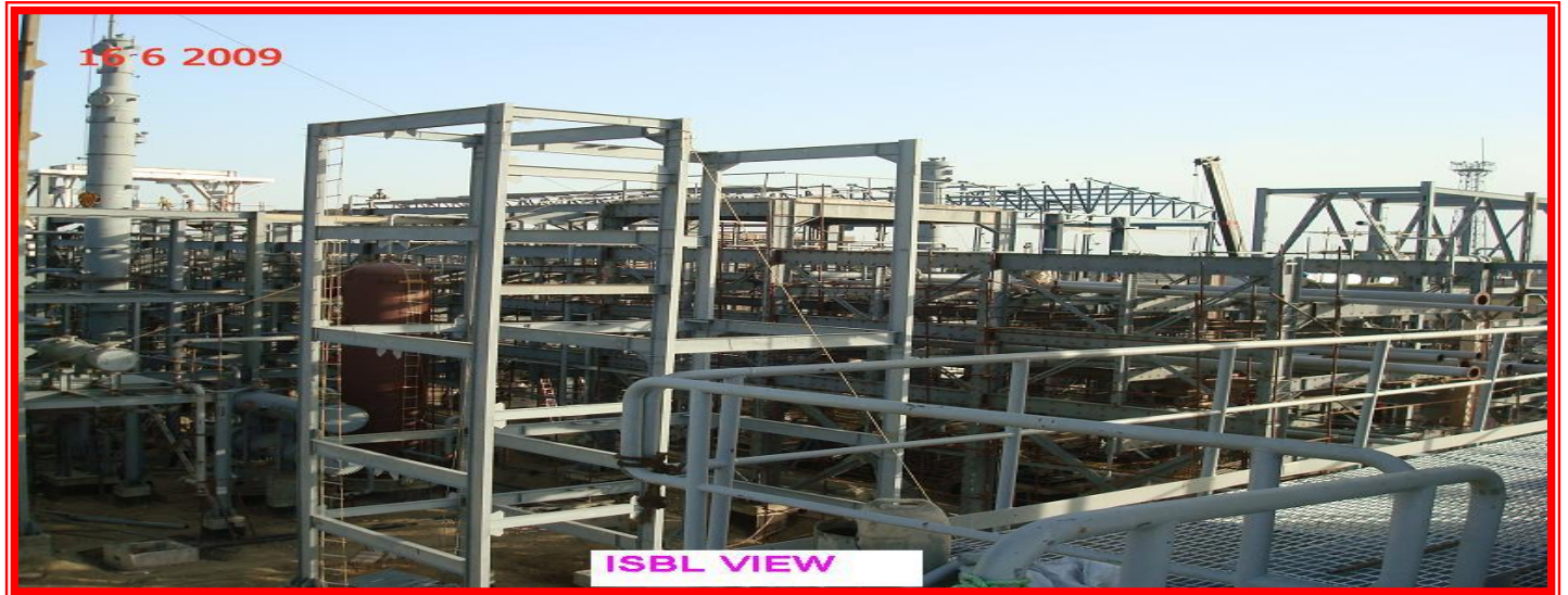
I.S.B.L. PIPING WORK DURING THE MSQ EURO IV PROJECT AT MATHURA REFINERY
